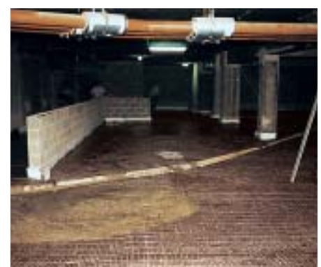
European Building, Brussels: The entire underground garage was put at risk by fluctuations in the groundwater level.
